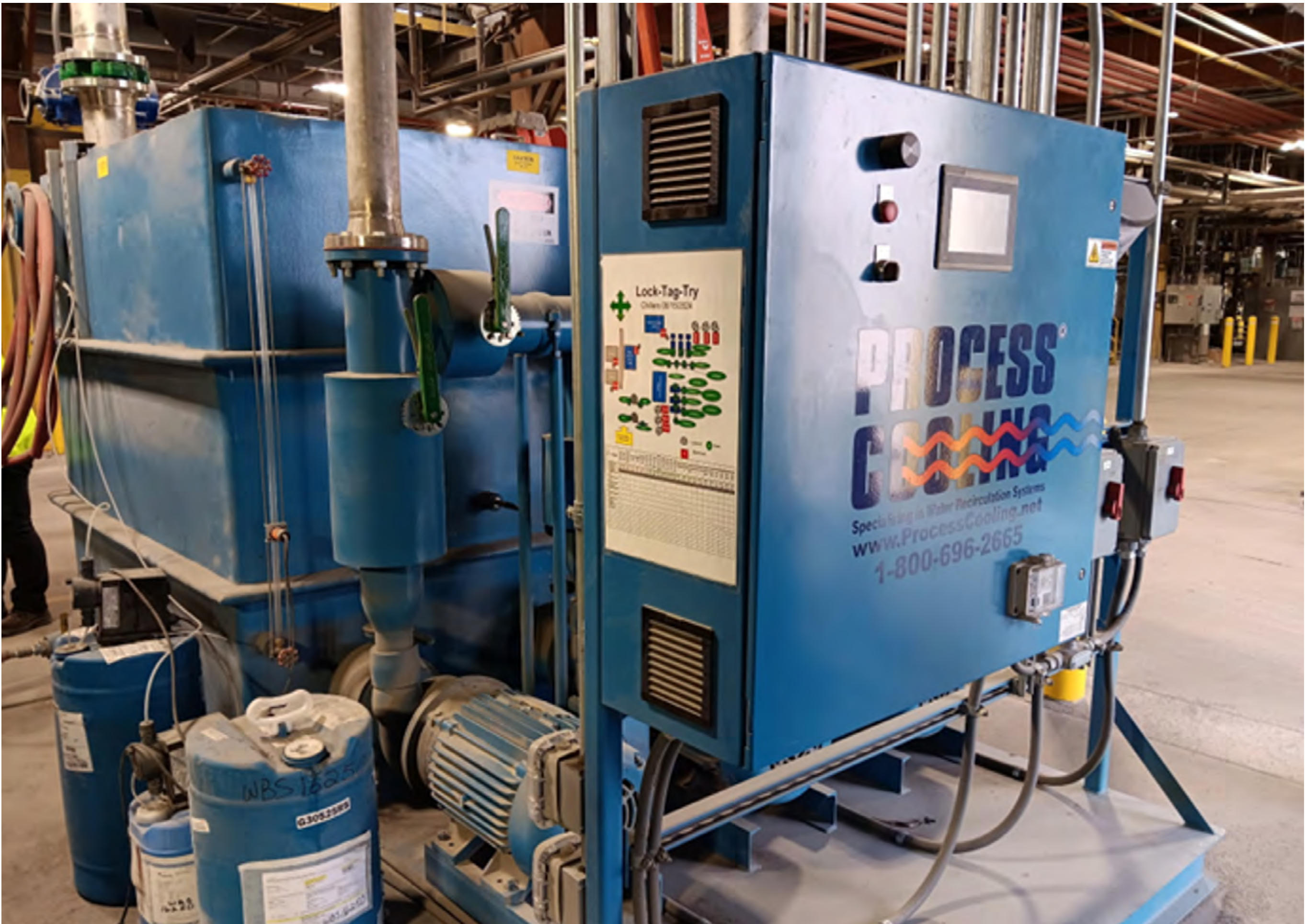
Photo submitted by: Michael Kennedy | Charlotte, North Carolina, U.S. A glycol chiller was installed for the drum cooling process at the Denver Roofing site.
